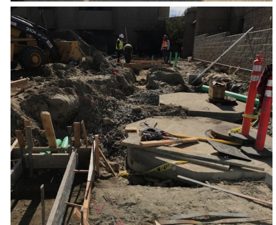
Stormwater Capture in the City of Duarte
